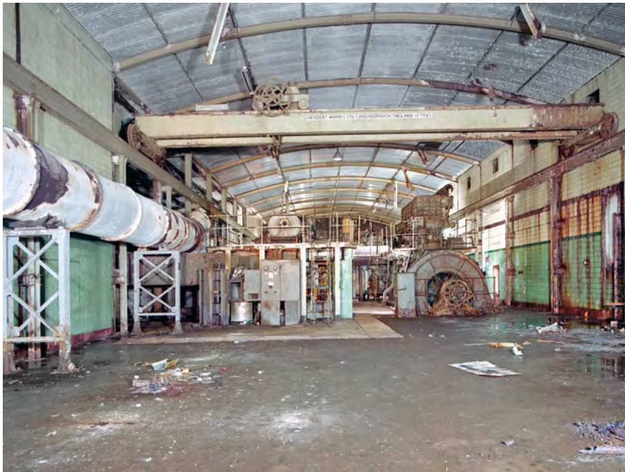
The massive underground generator hall at Calpe Hole. The two English Electric Fullagar diesel engines and generator sets are seen at the back of the hall.
